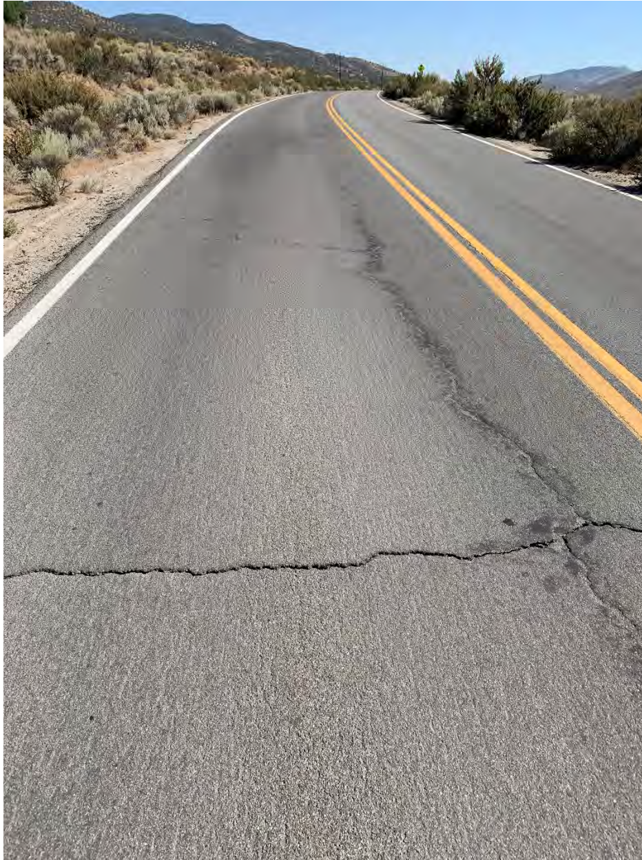
Figure 4. Pavement in Fair condition category (PCI 70-56).
