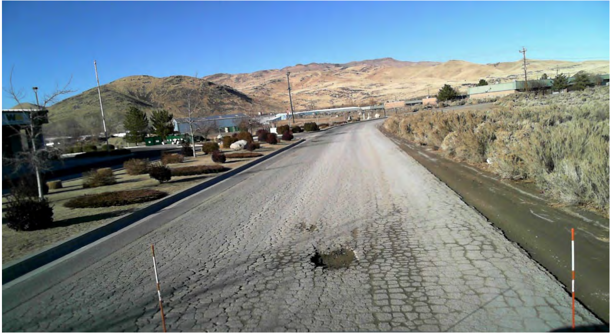
Figure 8. Pavement in Failed condition category (PCI 10-0).
