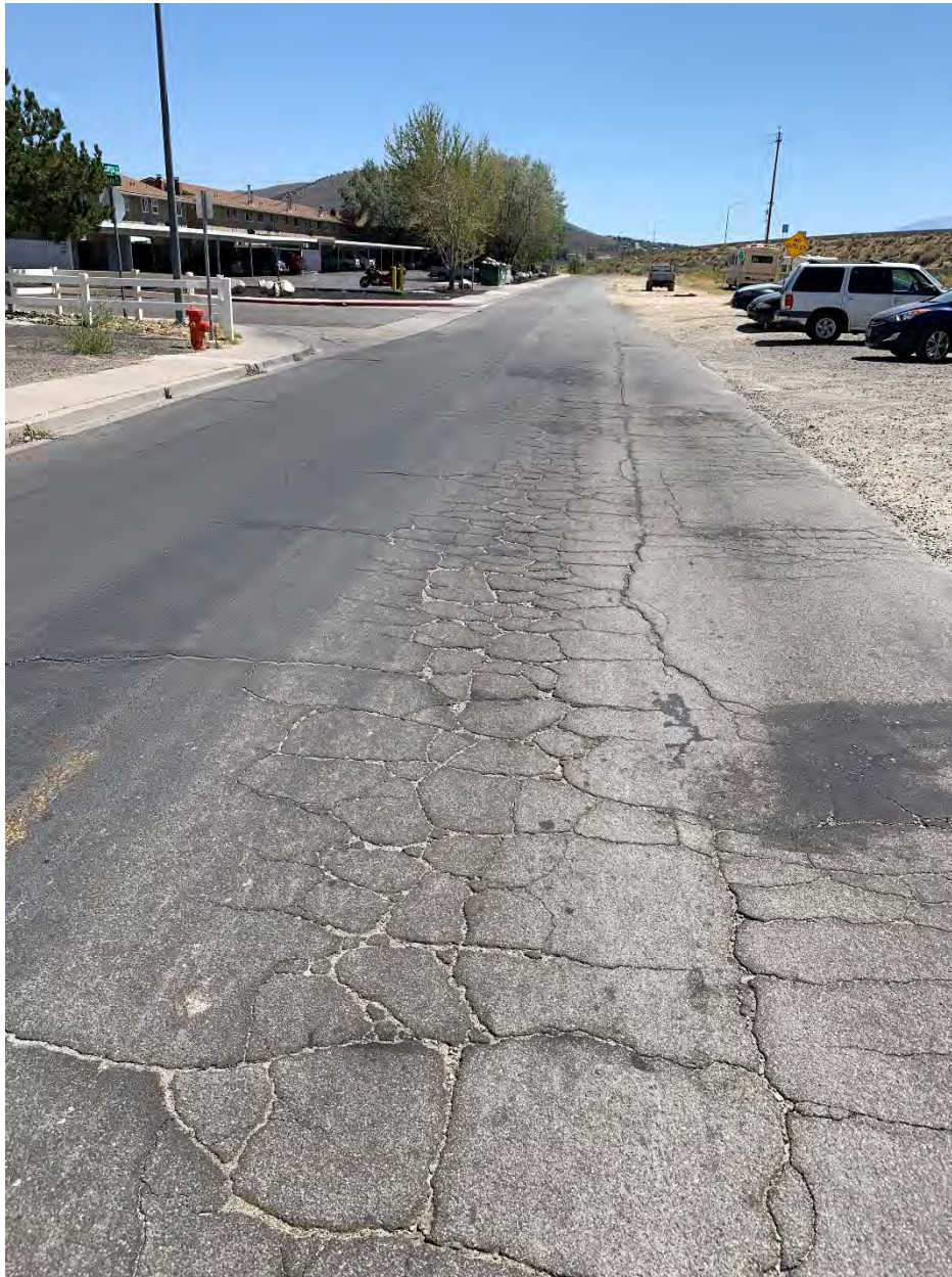
Figure 6. Pavement in Very Poor condition category (PCI 40-26).
